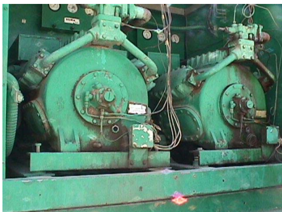
Fig. 4. Chiller No. 4 with two compressors.
