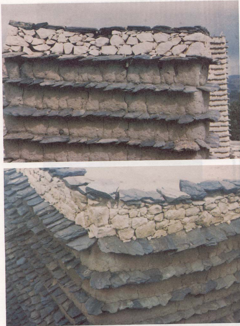
Fig. 6. Vertical exterior walls are topped with al-hayawa (stone course) that is used to withstand rain fall and protect mud courses.
