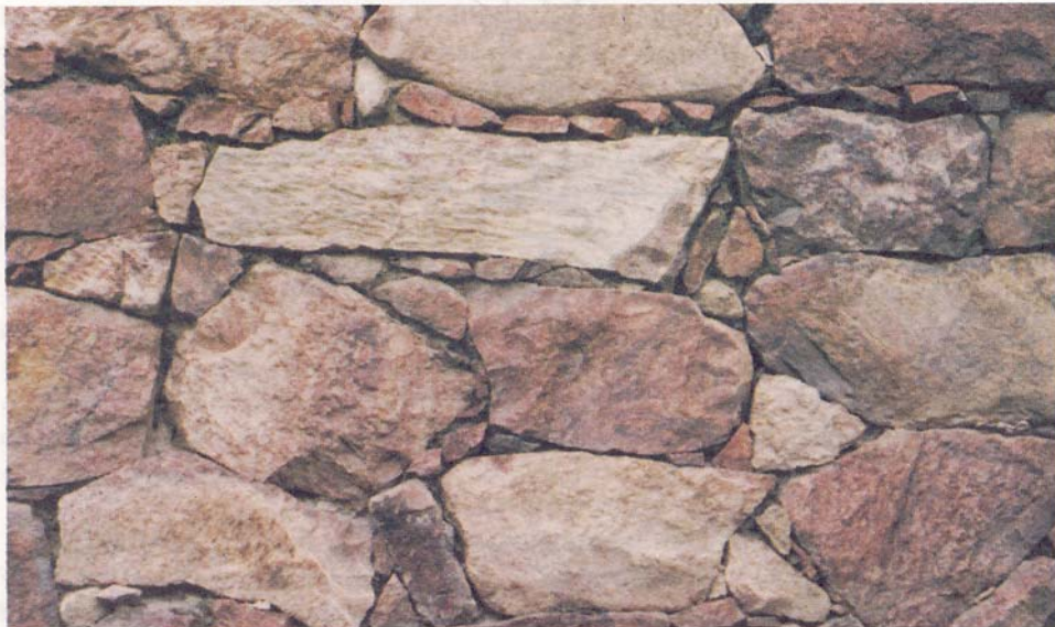
Fig. 4. Foundation walls are stone built starting often from a level about one meter below grade level and rising about 2-2.5 m. above ground level.
