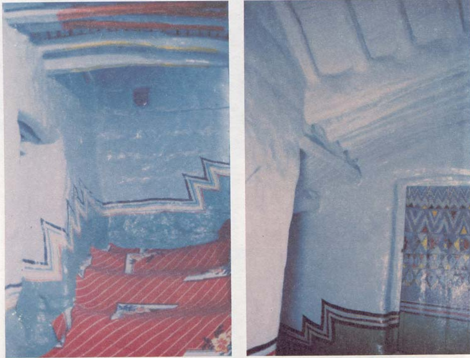
Fig. 14. Stair Construction Details. The staircase usually continues up unbroken from the bottom to the top of the house, a solid construction of adobe with a massive central stone and adobe pier, acting as a kind of structural spine to strengthen the whole building. The steps and the landing are of adobe built on top of wooden structural trimers and joists, and have steep goings.
