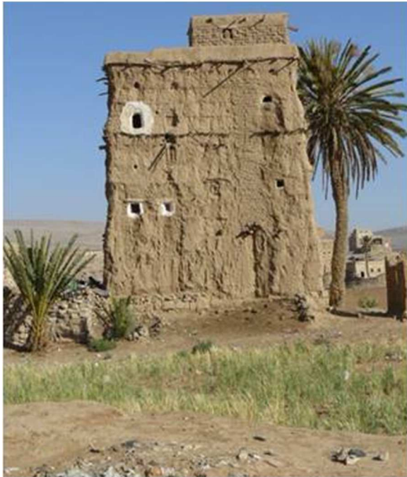
Fig. 3. A loam Building build by technique of Zabur in Maswarah - Marib, appearance of the affection of washing away of rainwater down the coated areas and in vertical shrinkage cracks severely due to the increasing of run-speed, March 2009.
