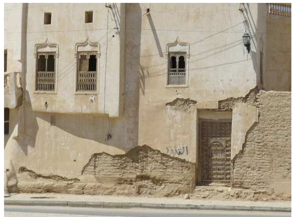
Fig. 5. Example of falling of lime plaster at the Palace of Hantoot - Tarim - Wadi Hadhramaut, March 2009.
