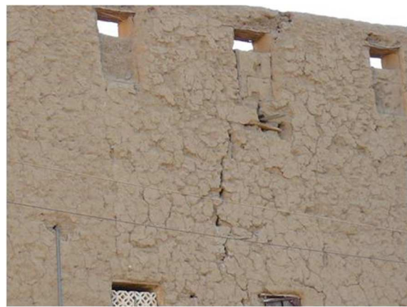
Fig. 2. A Residential building in Hisn, Al Ahmad- Wadi-Hadhramaut and show the severe effect of rain water on layer Al-Mahdhah, especially at the shrinkage cracks, March 2009.
